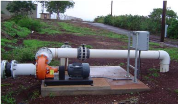
Newly installed pump-back station at Reservoir 225 in the Waiahole Irrigation System.
