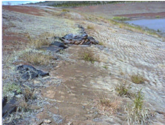
Damage lining, Bermuda grass, weeds and mulch.
