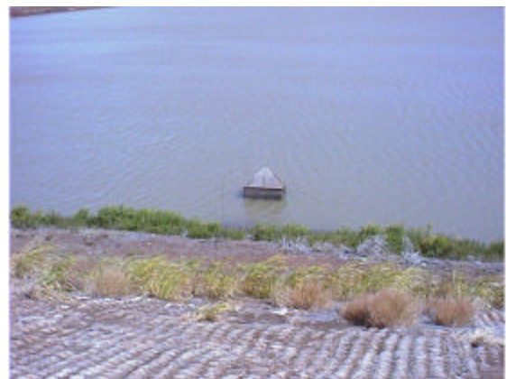
Outlet with screen leading to the distribution system.
