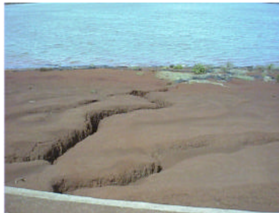
Soil erosion of the reservoir bank.
