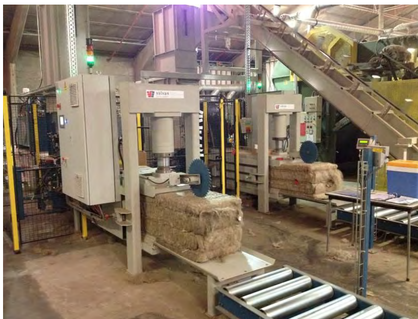
Picture showing 2 baling presses next to each other
